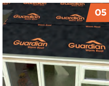
05 Breathable waterproof membrane is laid over the ply-wood and secured in place.
